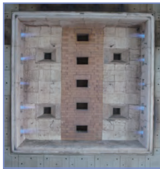
수직가열로A Vertical heating furnace A
