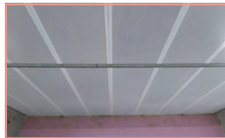
천장재 차음실 Room with sound-insulated ceiling material
